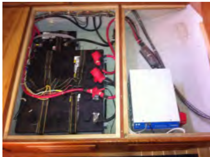
AGM Batteries (left) and the Xantrex Charger/Inverter (right)
